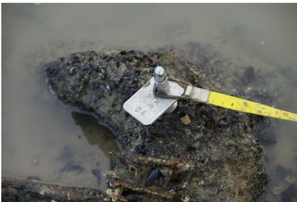
Figure 2 Tag number 4 (MiM 04) mounted in a wooden pile.
